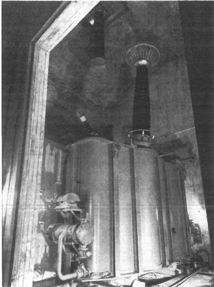
One of the four one-phase transformers in the large hydro-electric installation at Harsprånget. The transformer units each have a capacity of 115,000 kW at the transformation 16,000/380,000 k and are the first in the world with such high tension for commercial use. Photo: State Power Board.
